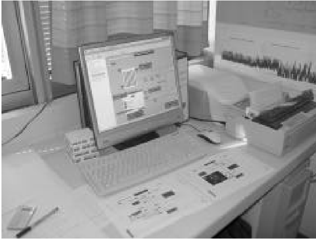
Figure 11. Central control system.
