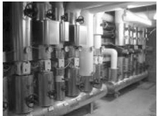
Figure 10. Warm water distributor.
