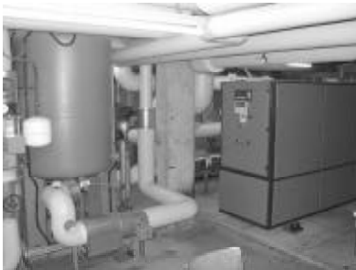
Figure 7. Absorption heat pump (left), and cogeneration equipment (right) .
