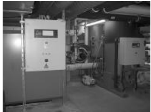
Figure 8. Gas fired condensing boiler (left) and absorption heat pump (right).
